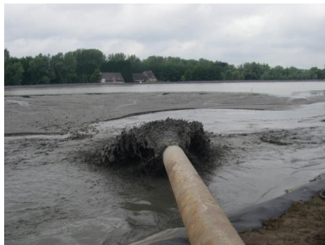
Figure 4: outlet of pipeline in lagooning area (temporary sand stock) along the Durme
