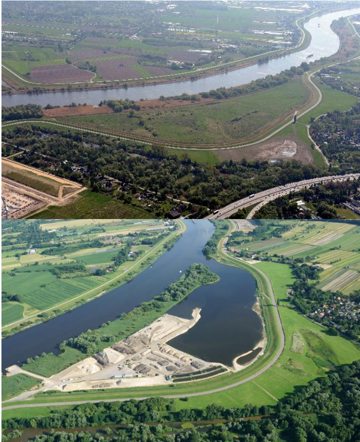
Figure 5a and b. The area of “Kreditsand/Spadenlander Busch” before the start of the works (©HPA) and in during the works in 2017 (© Holger Weitzel)
