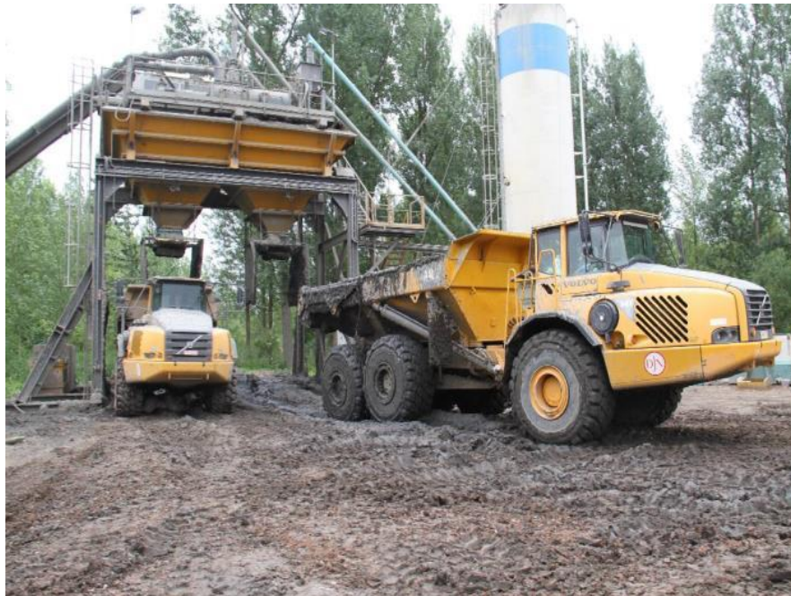
Figure 10: Example of a mobile treatment plant (Vlassenbroek)
