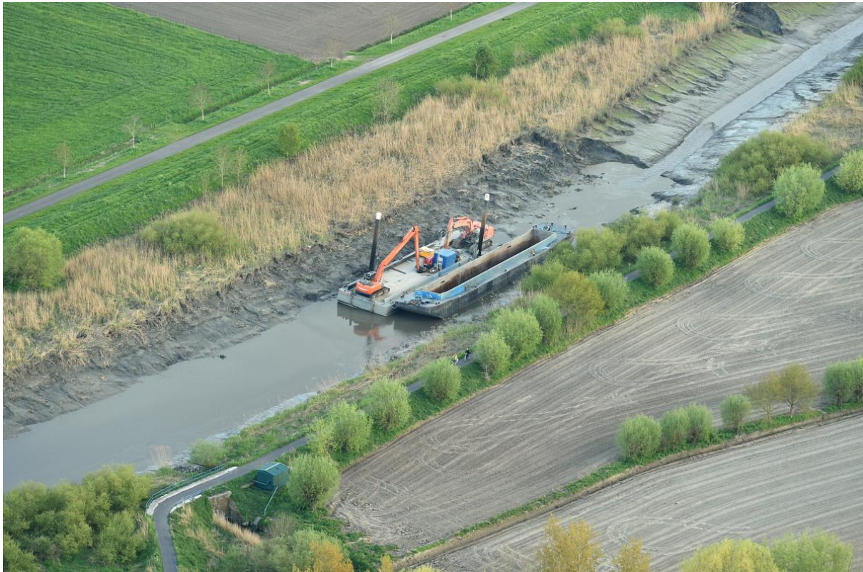
Figure 5: Hydraulic crane on a pontoon, with a barge, during low tide – Central part of the Durme
