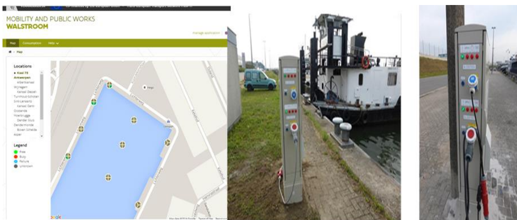
Figure 2. Shore power installations (low voltage) at quay 75 in Port of Antwerp
