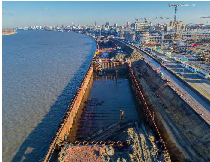
Figure 10: View of the first (left) and second (right) construction pit (source: Braincube commissioned by DVW)
