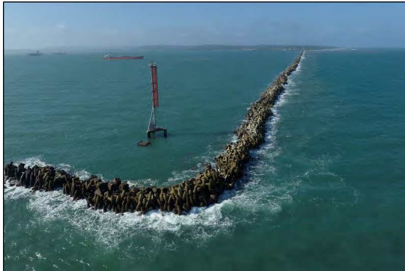
Figure 19: Aerial view of the West section of the breakwater where most damages are reported
