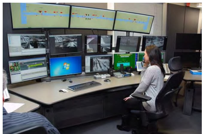
Figure 9: Remote Operations of Locks and Bridges
