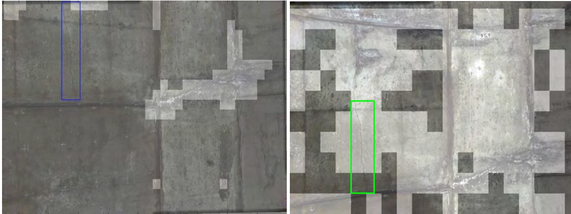
Figure 22: Defect detection (light areas) in concrete tunnel images. Example of a non-detected crack (blue box, left image). The same crack is detected using a more specific training (green box, right image) at the expense of a high rate of false alarms.
