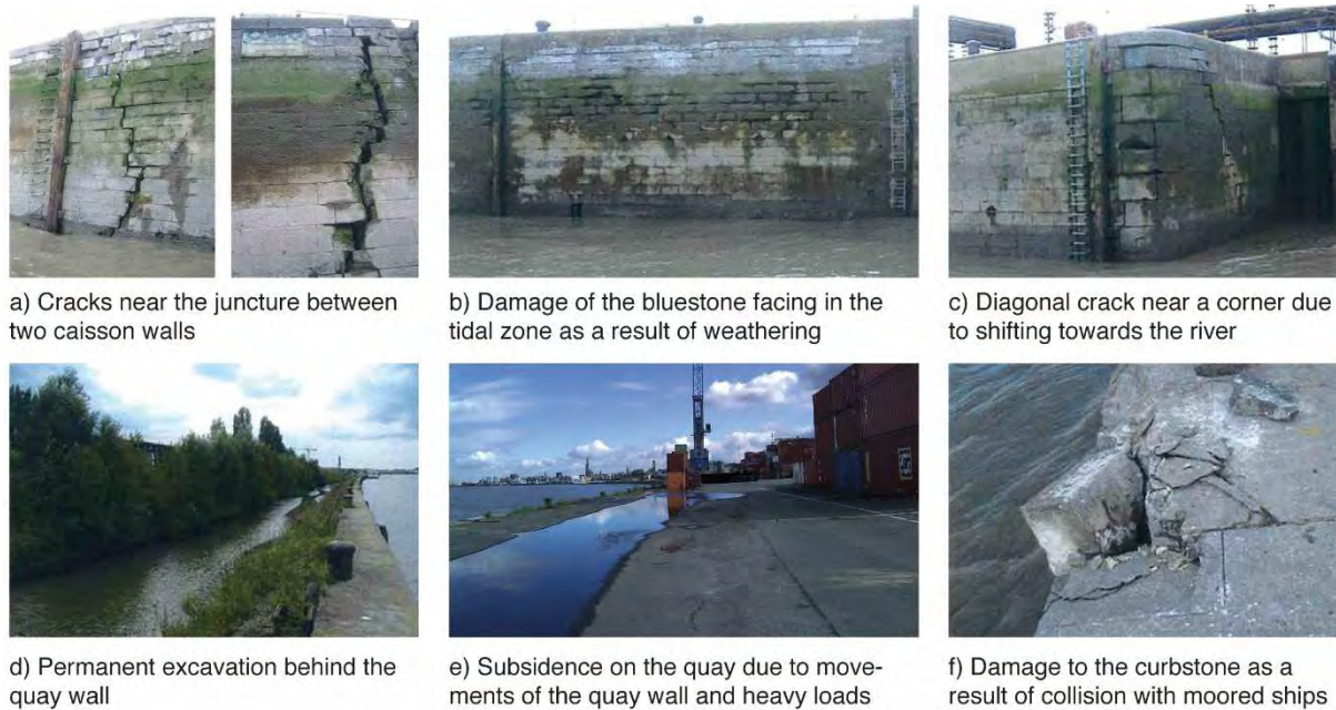
Figure 4: Inspection of damage phenomena on the Scheldt quay walls
