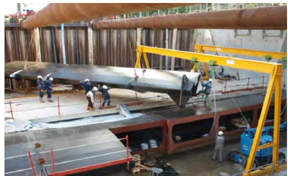
Figure 14 : Vives Eaux - gate lifted
