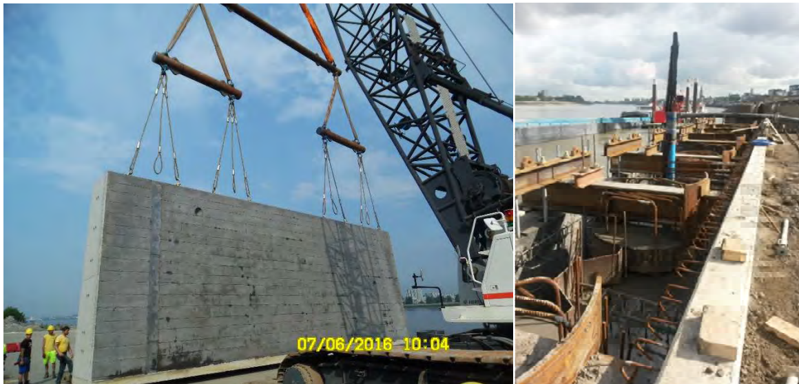
Figure 11: Prefabricated concrete facing elements of the front wall with interconnection holes, ready for placement (left) and elements mounted on the combined wall (right)
