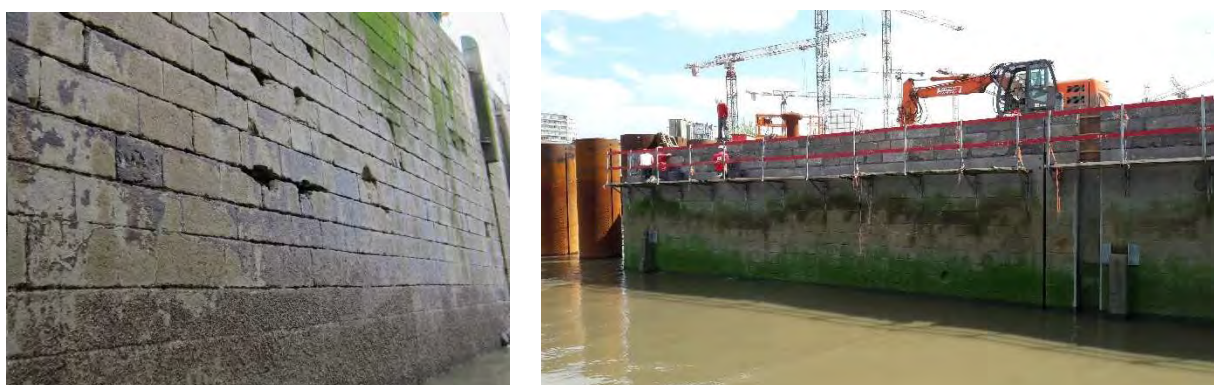
Figure 8: Original bluestone facing (left) and new concrete molded formwork with on top three rows of reused blue stone blocks (right)
