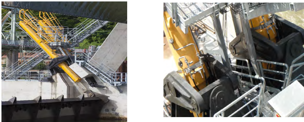
Figure 13 Hydraulic cylinders - vents downstream of the gate - cardans joints
