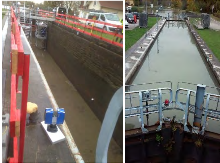
Figure 2: View of the empty lock during the TLS surveying (left) and the lock after refilling during the MSS surveying (right)
