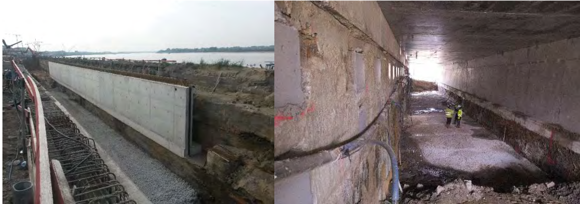
Figure 16: View of the chamber front wall placed on the existing quay wall (left) and view inside the stress relieving chamber (right)
