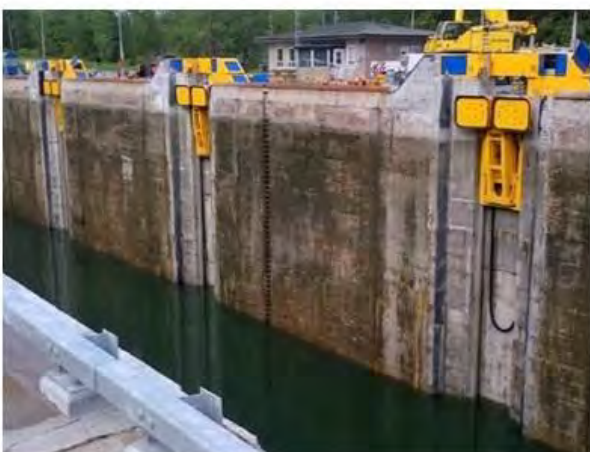
Figure 4: Three double units recessed in a lock wall
