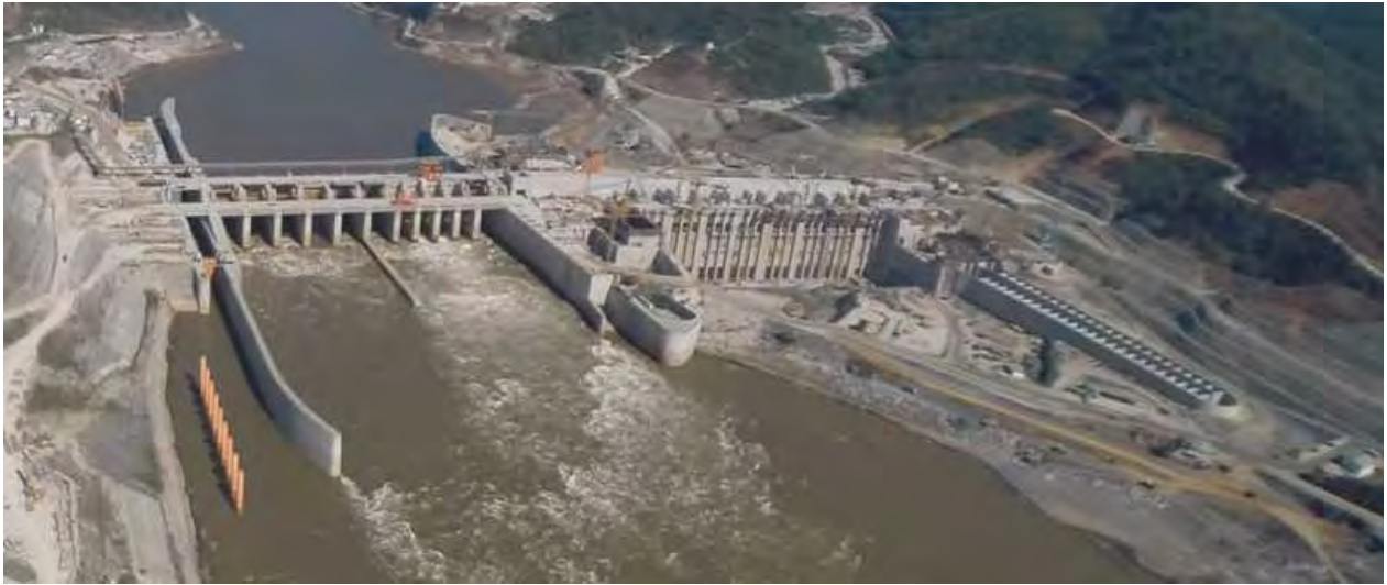
Fig. 2. General overview of progress of work as of January 2018 (photo: Marie Keller) From left to right: lock, spillway, low level outlet, intermediate block, power house and fish facilities
