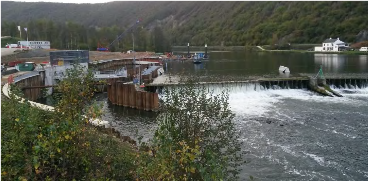
Lock 51 Saint Joseph. New channel for hydro power and fish pass on the left with the existing stake weir still in place during the construction phase.
