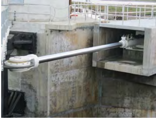
Fig. 9: Large Cylinder operating a miter gate
