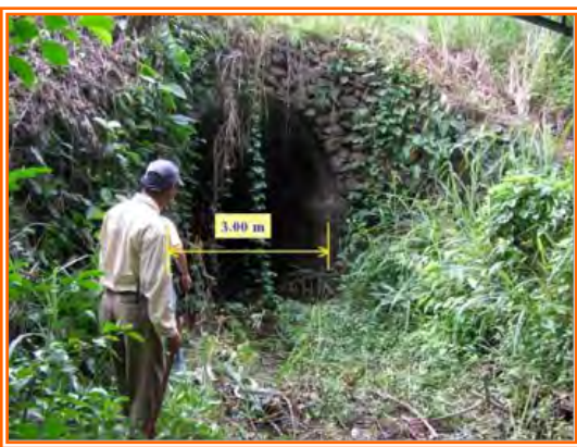
Figure 5. Horseshoe culvert in the Victoria Norte creek the Brujas road. View from upstream in the channel of the gulch. Dimensions 3.00 x 3.00 m. JACM / June 2007
