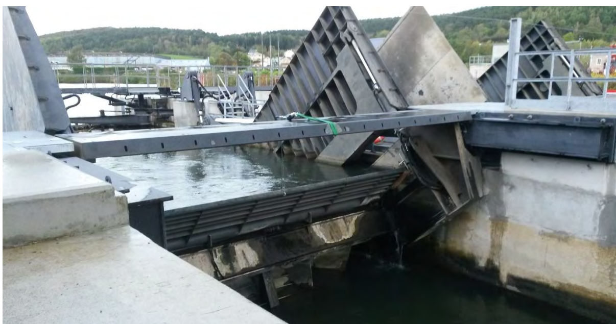
Lock 57, Ham. Very Low Head turbines in operation. In times of flood, the turbines are lowered down and the doors are closed over the turbines to allow the full area to be used for flood discharge
