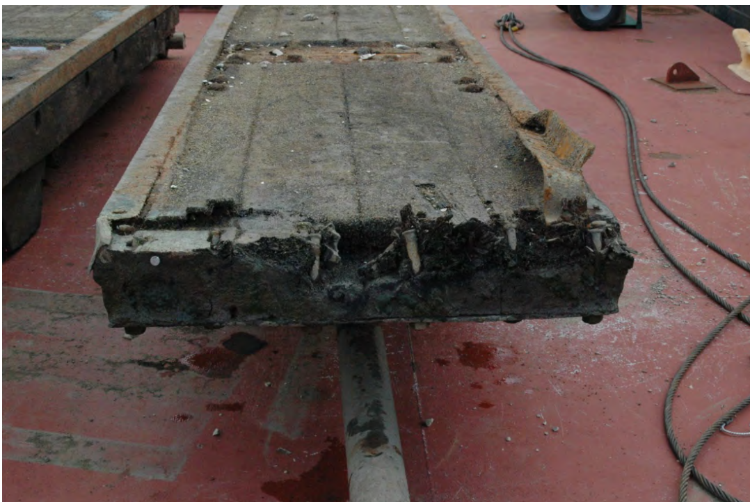
Figure 4: Deteriorated Timber Wicket Gate
