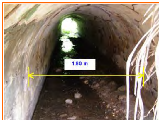
Figure 6. Horseshoe culvert in the Victoria Sur gorge, on the Brujas road. View from downstream in the channel of the gulch. Dimensions 1.80 x 1.80 m. JACM.
