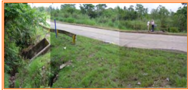
Figure 4. Culvert concrete drainage system 3.00 x 3.00 on the road to Brujas, which will have to be removed to run the diversion channel of the Cocolí river. JACM / June 2007
