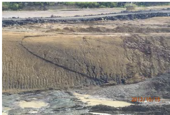
Figure 6. Example failure of outboard core trench slope
