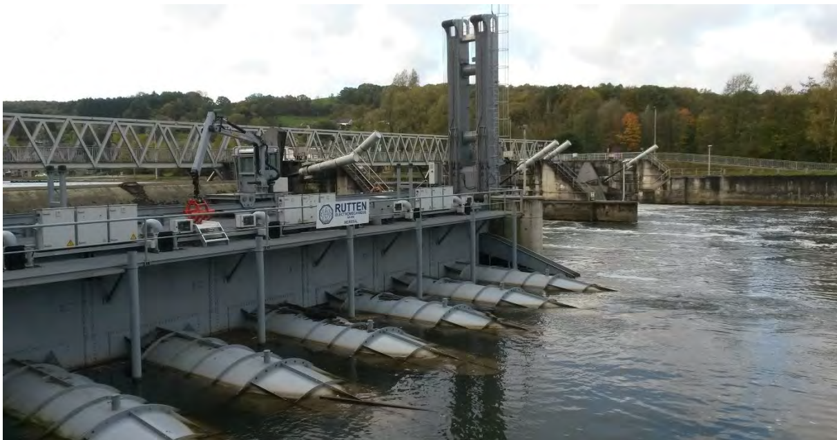
Lock 1 Hastiere showing six turbines mounted on a steel deck immediately in downstream of the weir gates. The vertical tower is part of the lifting equipment that lifts the deck clear of the river in times of flood.
