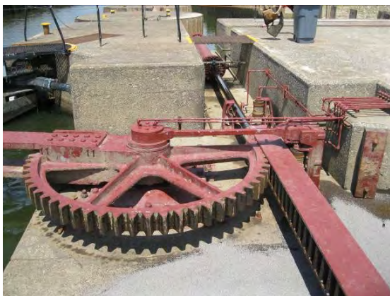
Fig. 5: Ohio River Linkage with rack gear and sector gear
