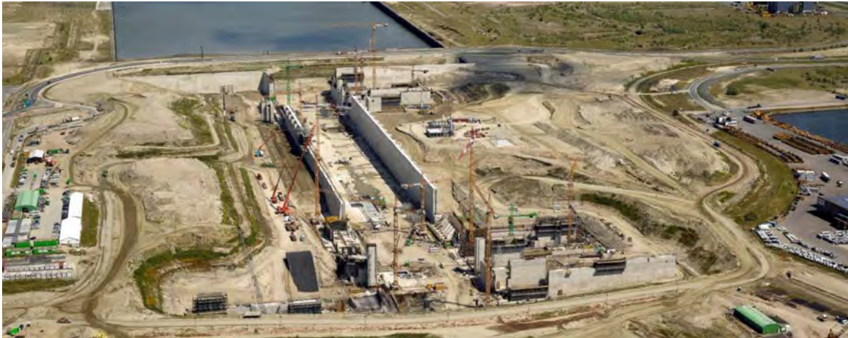
Figure 13. Construction of Kieldrechtsluis in Antwerp by means of a dry construction method.
