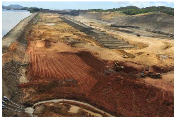
Figure 5. Dam 1E foundation with cellular cofferdam (left), PAC excavation (right), and rockfill shell on the inboard dam foundation
