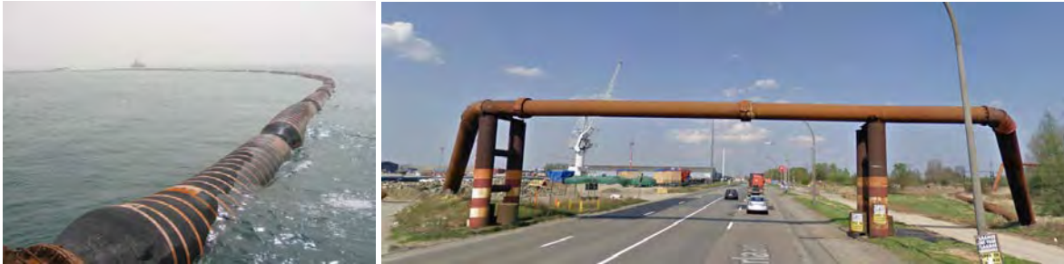
Figure 11. Floating pipe line and bridge construction of land lines over a road.
