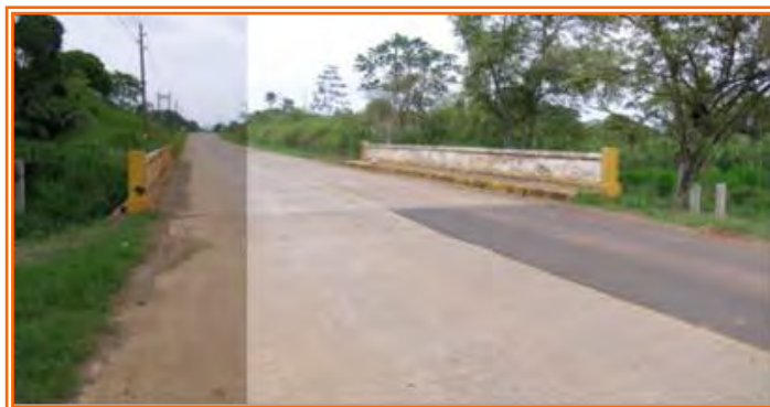
Figure 7. View of the bridge over the Velázquez River, on the Brujas road looking towards Cocolí. JACM.
