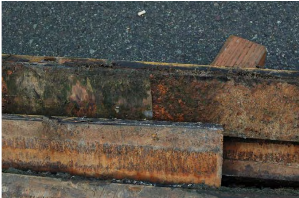
Figure 1: Corroded and Abraded Carbon Steel Miter Blocks
