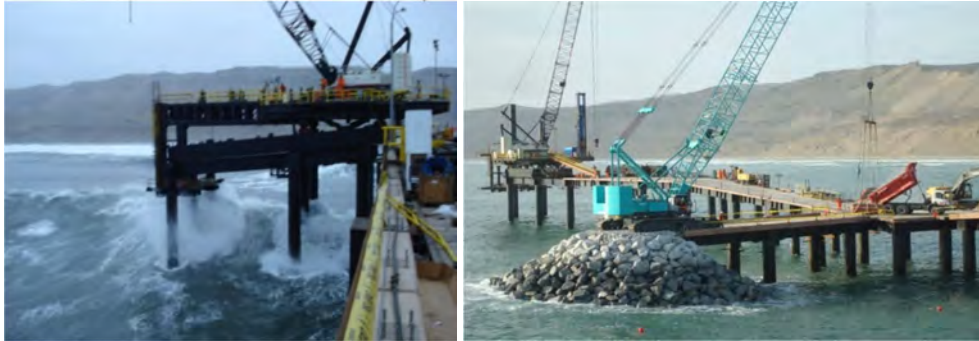
Figure 15: Rock Load Out Facility - RLOF - Melchorita Peru
