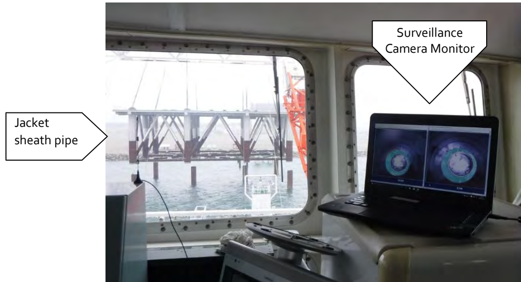
Figure 5: Jacket Induction with the help of surveillance camera
