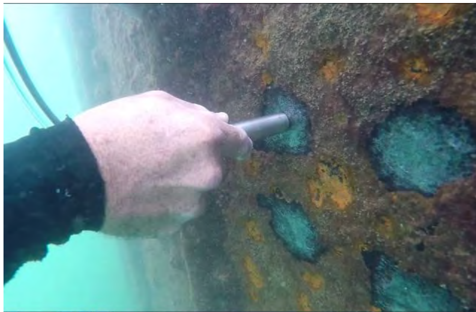
Fig. 3 Underwater Procedures at the Marina in Quepos (Above) Cleaning of measurement points (Below) Thicknesses measurement with ultrasonic sensor.
