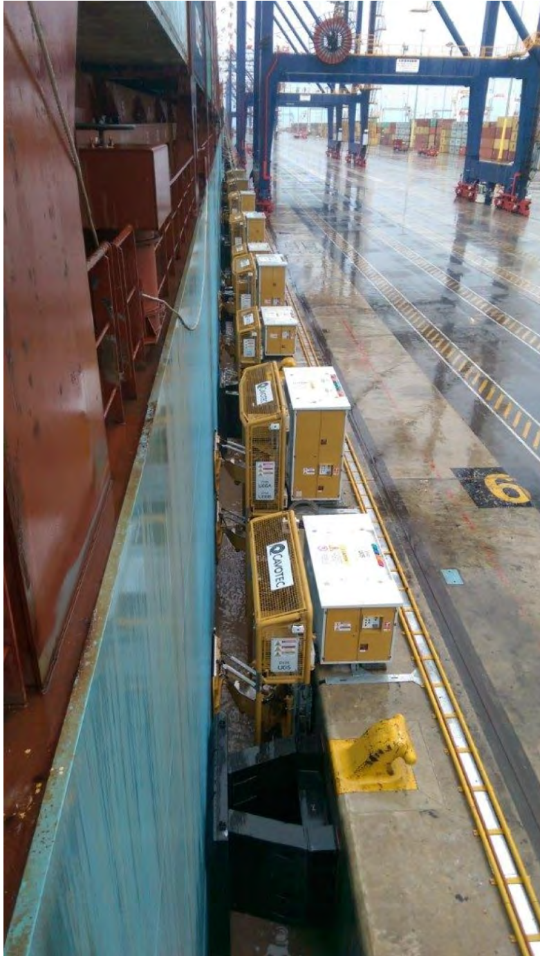
Cavotec MoorMaster™ MM200C17 system installed in the Port of Ngqura
