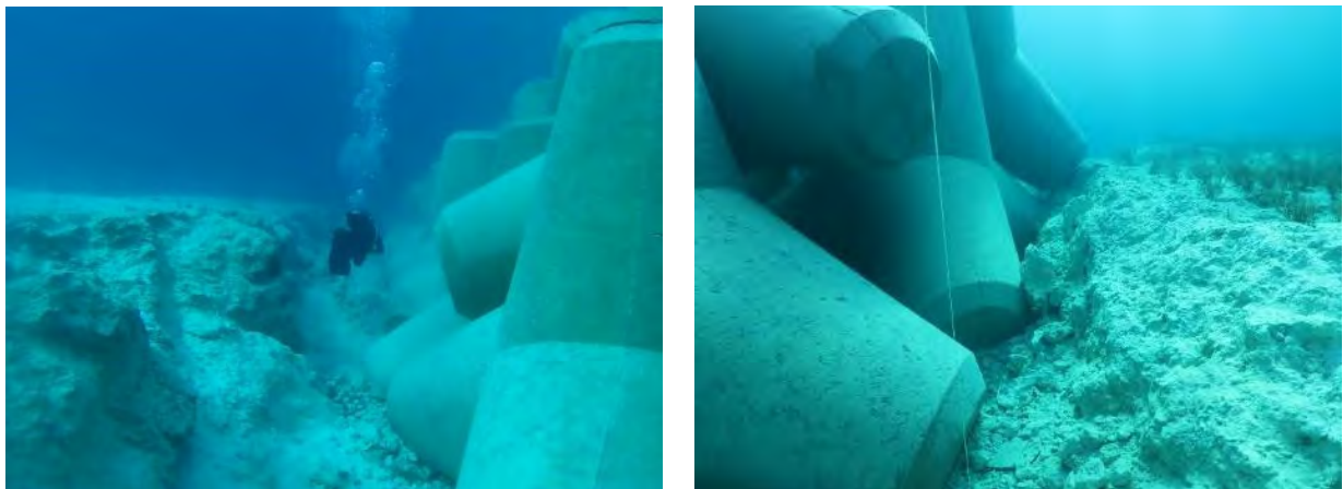
Figure 13. Prototype excavated trench and confinement of Tetrapods by the trench at the shallow section.
