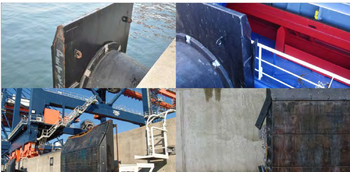
Figure 3: Damaged fender panels at Euromax Container Terminal Rotterdam (Photos PoR)
