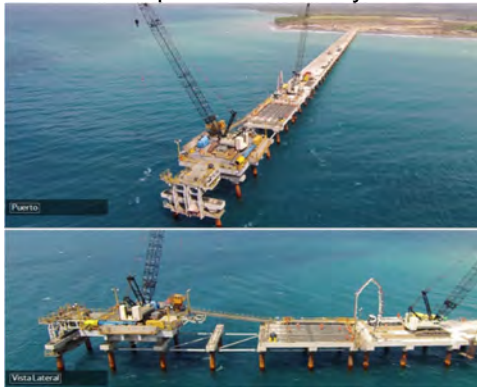
Figure 30: Import Coal Terminal - Punta Catalina – Dominican Republic
